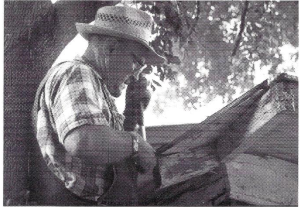
A "One Heart...Many Hands" volunteer repairs a roof at a project site.
